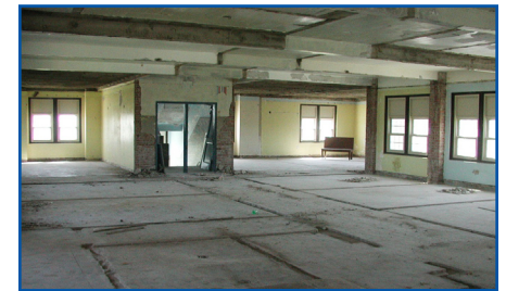
Biltz Hall second floor interior completely removed to make ready for new walls, rooms, and furnishings.
